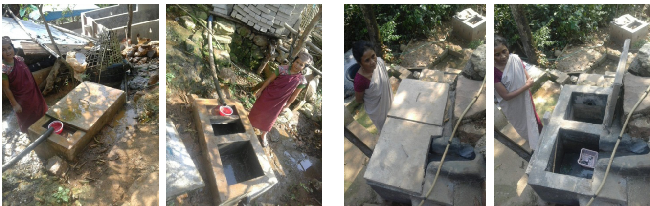
Kitchen Waste Water Soak Pit with Bio-Filter & Oil Trap Dymmiew & Massar Village, Pynursla C&RD Block, EKH
